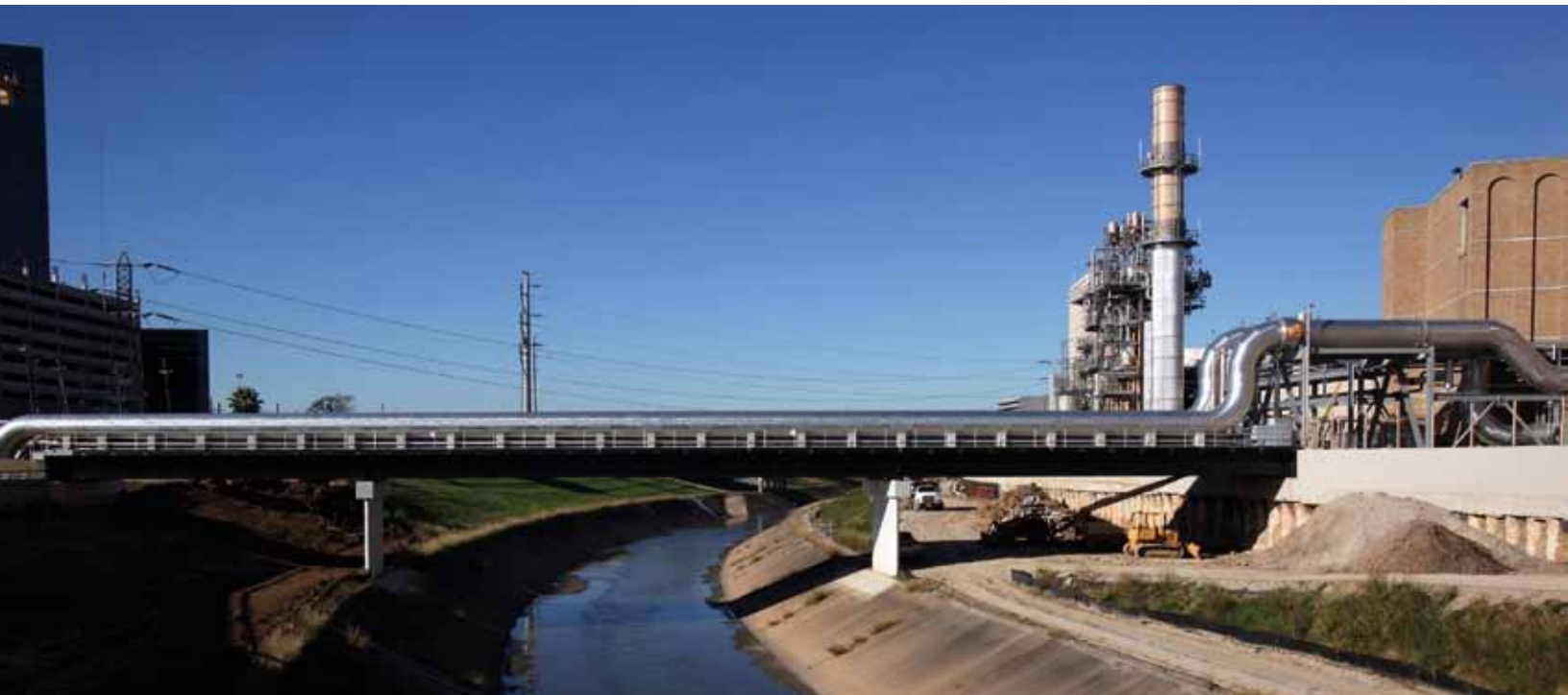
Figure 11: Pipes run over a canal at Thermal Energy Corporation, the district energy company that provides heating and cooling to the Texas Medical Center in Houston, the largest medical center campus in the world.
