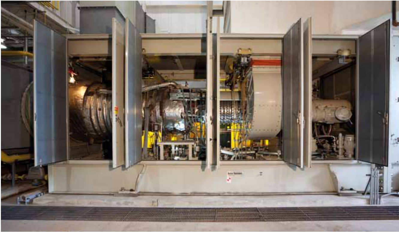
Figure 23: A Solar Turbines Titan 130 generator set provides district heating and electricity to London District Energy in London, Ontario, Canada.
