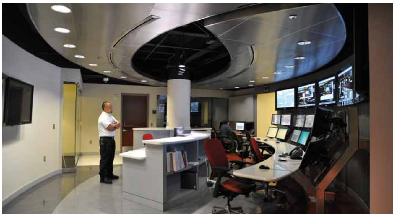
Figure 13: The control room of Thermal Energy Corporation in Houston, Texas, where a recent $377 million energy infrastructure expansion added 48 MW of CHP that operates at 80% efficiency.
